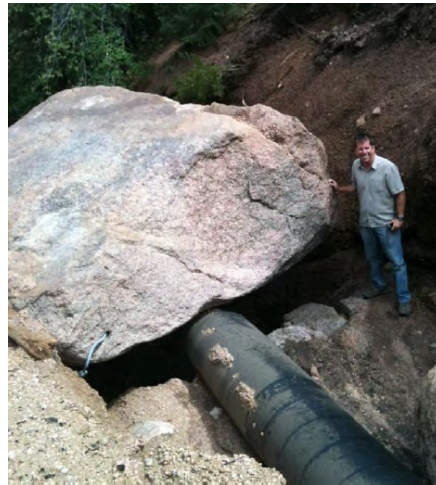
Exposed pipeline after the Colorado Springs 2012 Waldo Canyon wildfire
